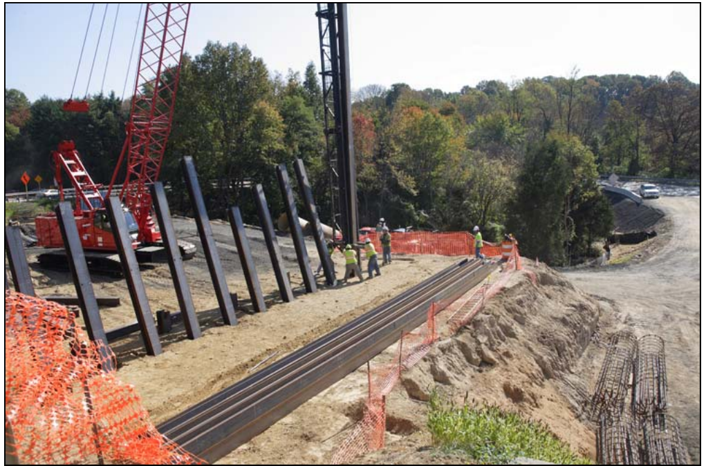
When old bridges are demolished, new ones will replace them. At the Little River Turnpike interchange crews drive piles as part of bridge construction at I-495.
