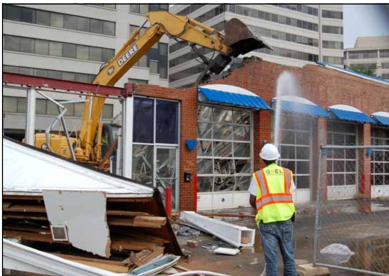
A worker sprays water to control dust at the old Merchant Tire, near the future location of Tysons Central 7 Station in Tysons Corner. Photo by Shea Daugherty, Dulles Transit Partners
