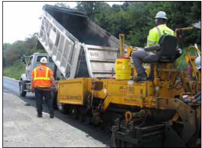
Paving crews lay down asphalt for the fourth lane of I-95. Photos by Mike Salmon, Virginia Megaprojects
